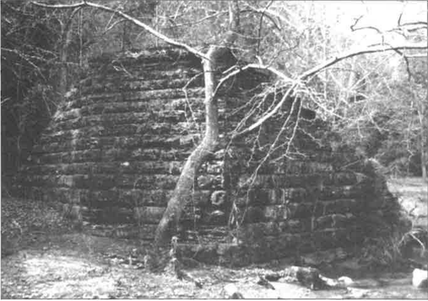
Above: Structure 2 (at 3560 on the bottom map on the previous page)—abutments for a forty-five-foot bridge over Broad Creek.
