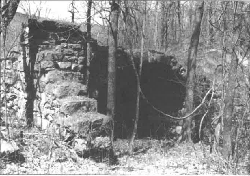
Above: Structure 6 (at 3770 on the map at the top of the previous page)—incomplete twenty-foot arch on Broad Creek at Rt. 610 (Plank Road).
