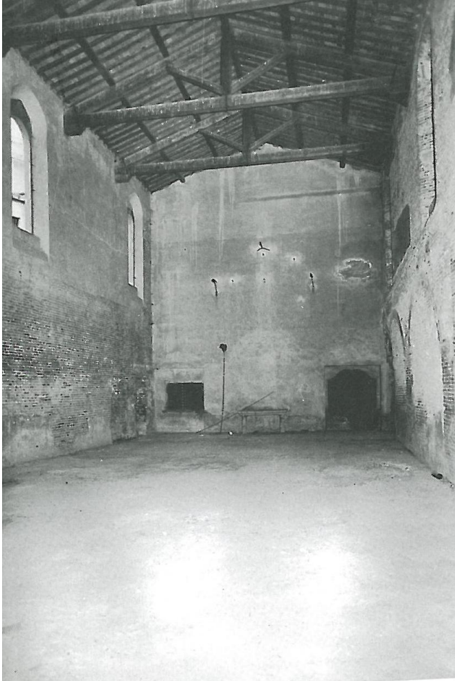
Figure 7. Interior of Nuns' Choir of San Domenico, c. 1990's, to the West.
