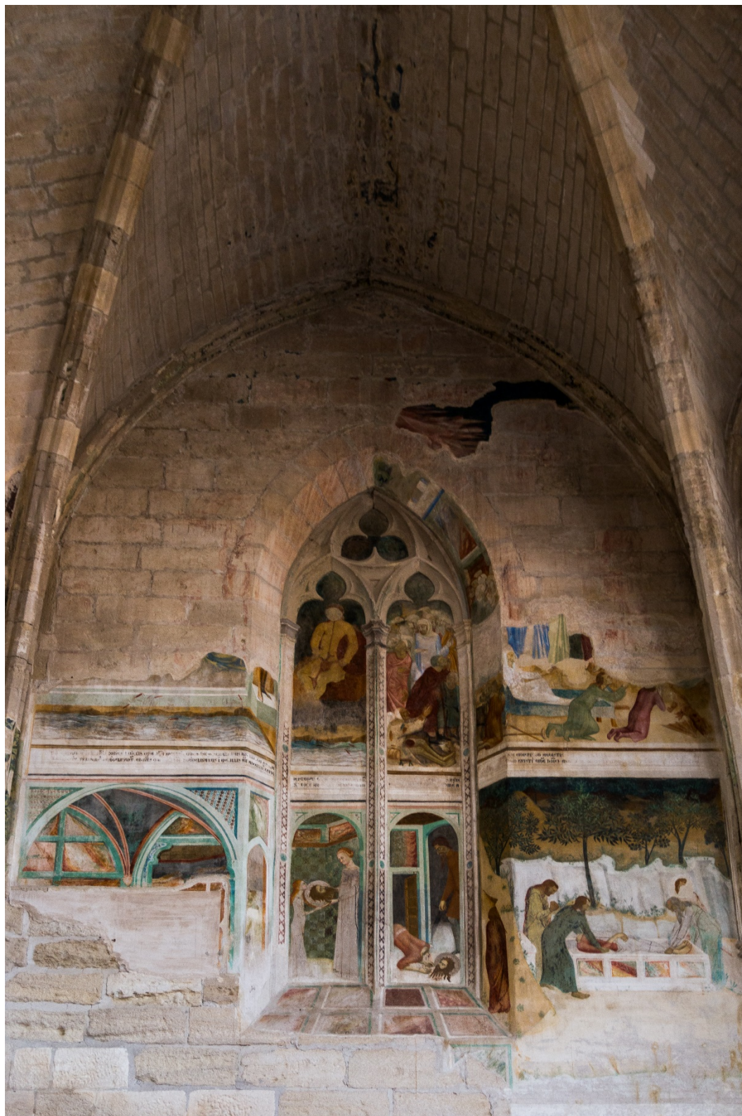
Figure 19: Detail of the western wall of the chapel showing degradation of the fresco cycle
