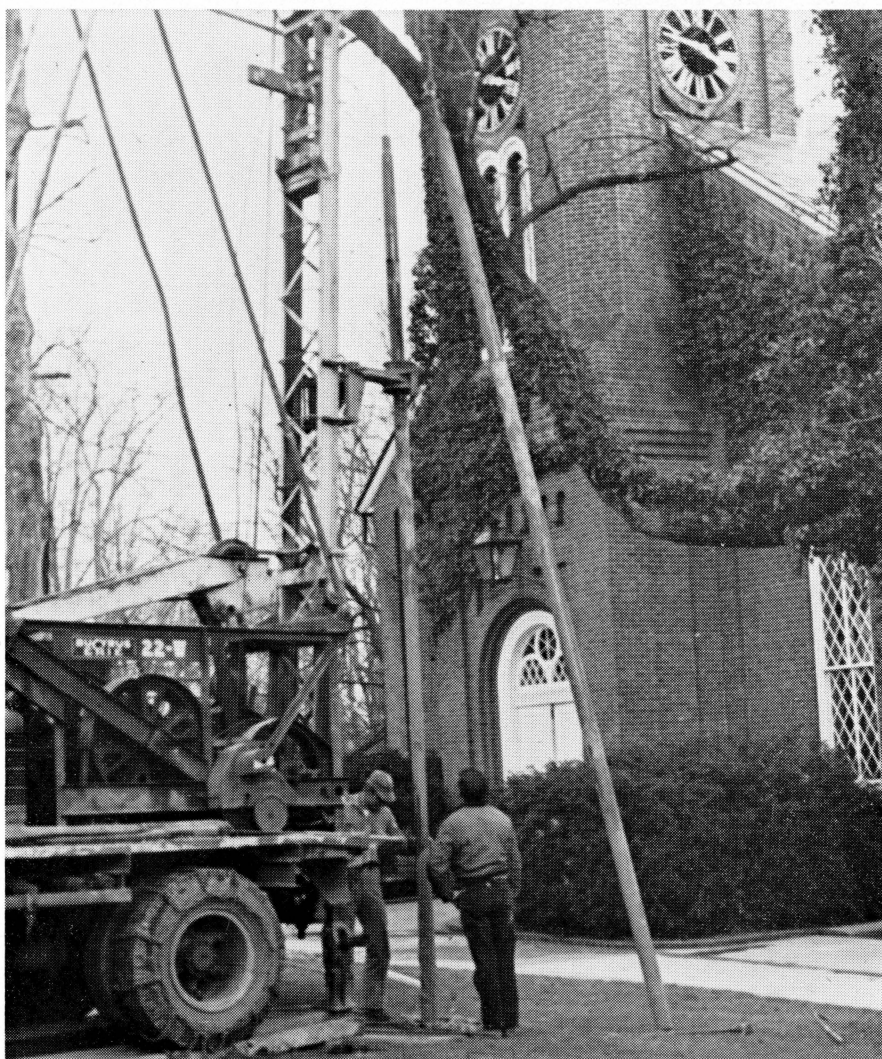
A well-digging apparatus tests for rock near Lee Chapel in preparation for necessary forthcoming excavations.
