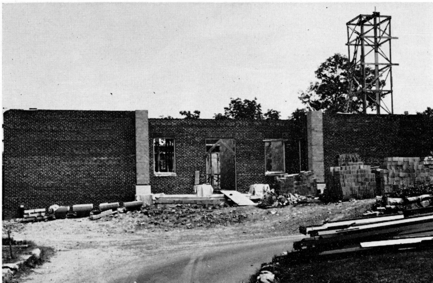
Delay in the shipment of steel brought work on the new academic building to a temporary halt in July. Work has now been resumed, and plans call for occupancy by January.
