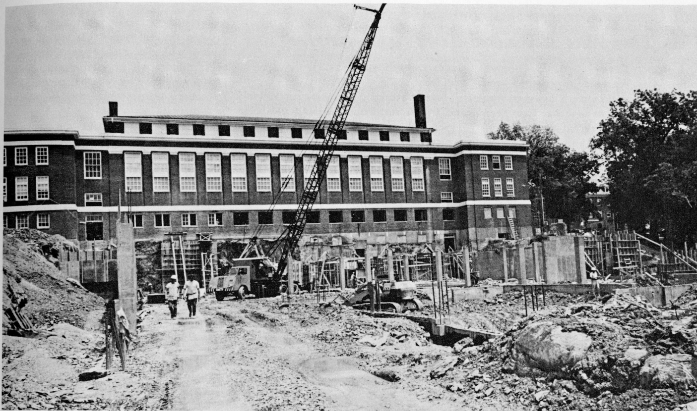
Doremus addition extends from rear of old building to house new swimming pool, handball and squash courts, and new basketball arena.
