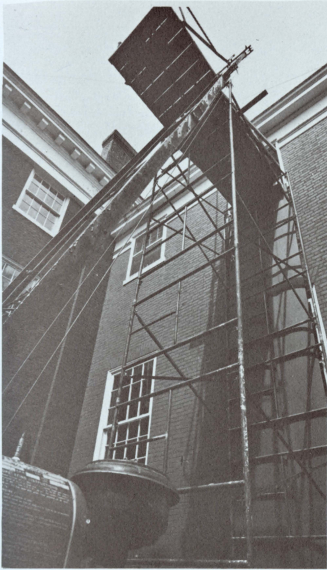
Scaffolding is outward sign of physical changes occurring inside the Law School building.
