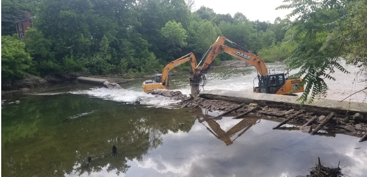
Figure 2. Image of the Jordan's Point Dam being removed in May 2019. Timbers of the older, un-breached crib dam in front of which the concrete dam was built are visible.
