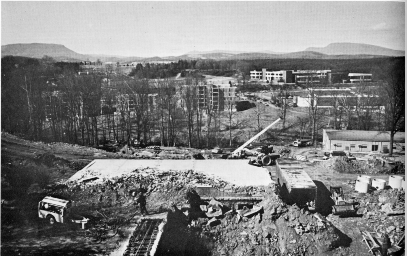
This picture, made through a screened window in the rear of Washington Hall, shows much of the major construction associated with the development program: Lewis Hall (top right); Woods Creek Apartments (left); heating-cooling plant (center right); and construction on the new undergraduate library (foreground).
