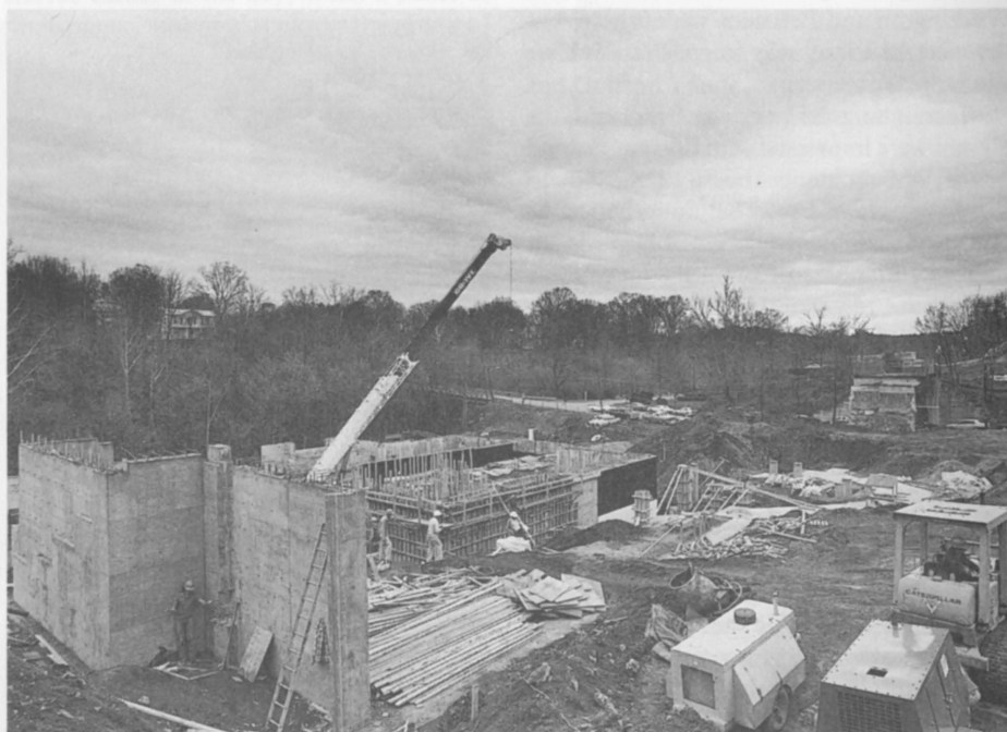
Construction is proceeding on schedule for the Lenfest Center for the Performing Arts.
