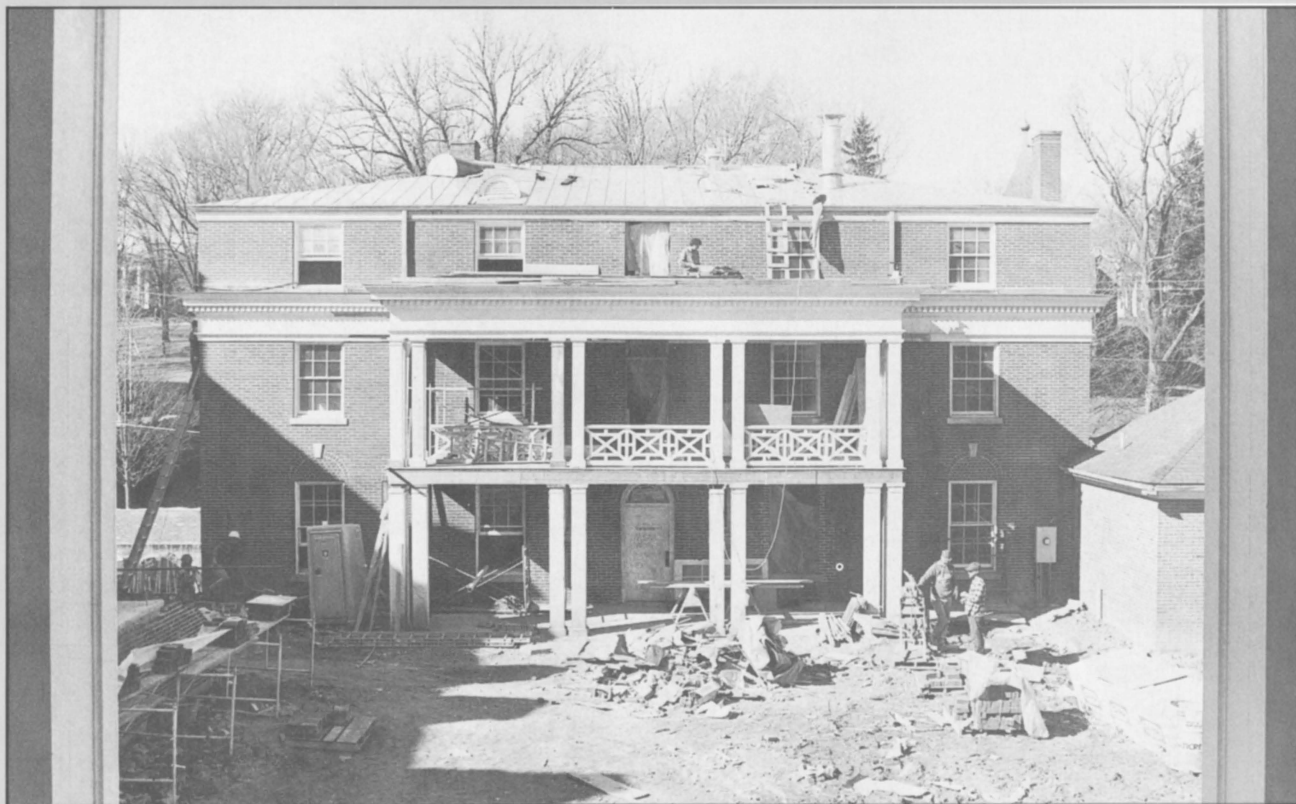
Above, workers build a wall near Beta Theta Pi. Below, the windows of Pi Kappa Alpha show a clear view of construction at Beta.
