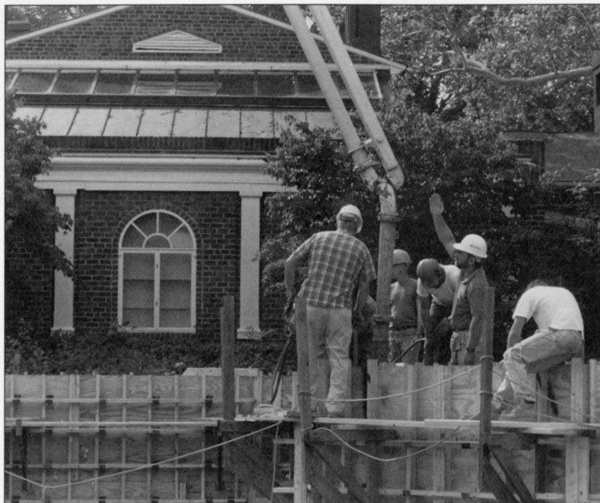
A view of the construction work being done on campus for the Watson Gallery.
