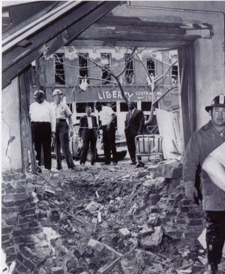
A DETONATION EQUAL TO 10 STICKS OF DYNAMITE BLEW A HOLE IN THE EAST WALL OF THE 16TH STREET BAPTIST CHURCH ON SEPT. 15, 1963. WINDOWS WERE BLOWN OUT IN THE BUILDING JUST BEHIND POLICE AND EMERGENCY WORKERS.
