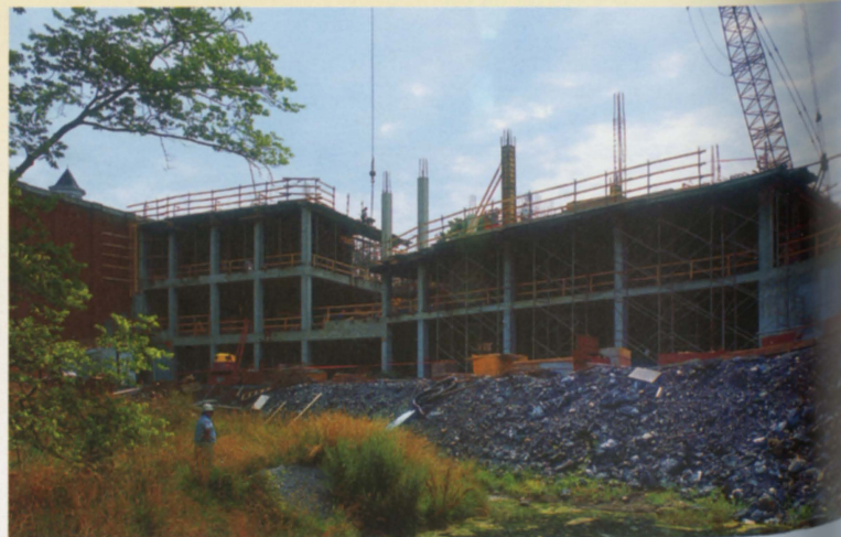
A VIEW FROM THE WOODS CREEK SIDE OF WILSON HALL. THE INCORPORATION OF GLASS ON THIS PART OF THE BUILDING WILL BRING NATURAL LIGHT INTO THE ART STUDIOS.
