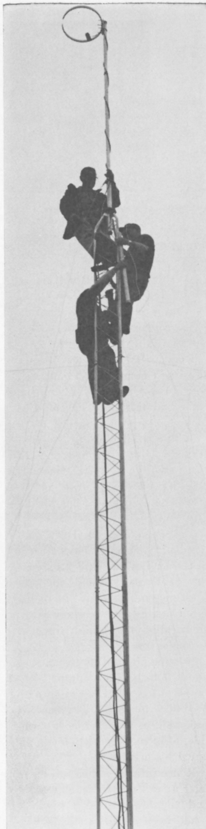
Workmen put the final touches on WLUR-FM's antenna above the roof of Reid Hall.
